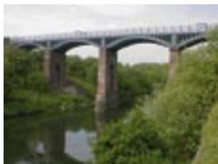
Outwood viaduct, Bury – a £1 million project to restore a 19th century railway viaduct as part of a country park trail within the National Cycle Network.
